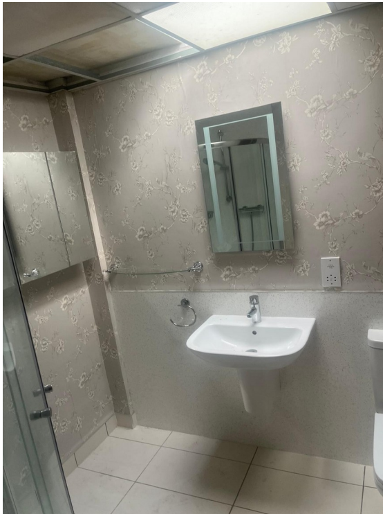
Before: dated sanitaryware and finishes.
